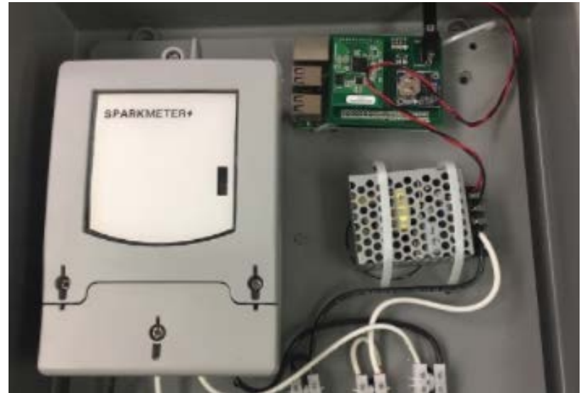
SparkMeter circuit controllers
